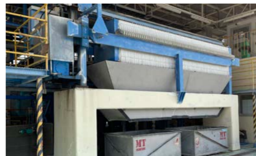
Automated backwashing disc filter equipment at TOTO (Thailand) Co., Ltd.
