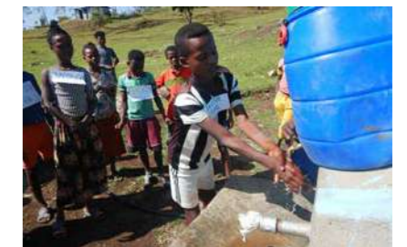
Installation of hand-washing station by TOTO Water Environment Fund grantee organization (Ethiopia)
