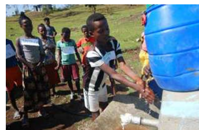
Installation of hand-washing station by TOTO Water Environment Fund grantee organization (Ethiopia)
