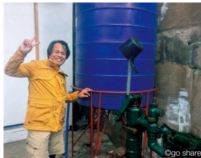
Water storage tank installed at Learning Center
